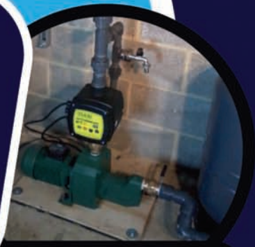
WATER SUPPLY PUMPS
